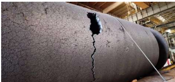
Full circumferential crack, coiler drum
